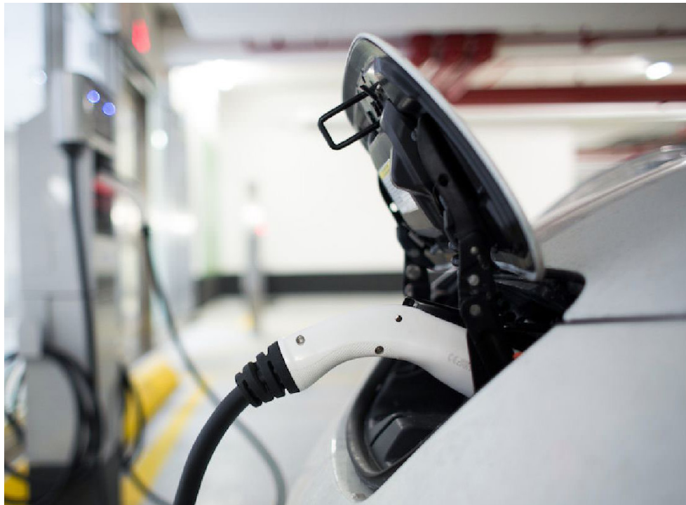
Electric vehicles are here to stay, says NOTL Hydro president Tim Curtis. He wants to make sure NOTL's hydro grid can support the demand for more power. SUPPLIED
