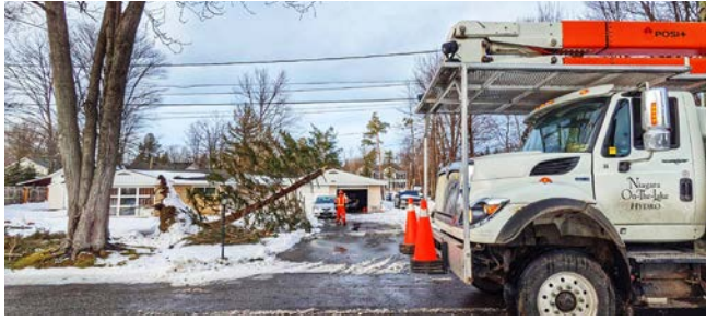
Line workers from NOTL Hydro spent a chunk of the holiday season cleaning up Fort Erie after a major storm. SUPPLIED
