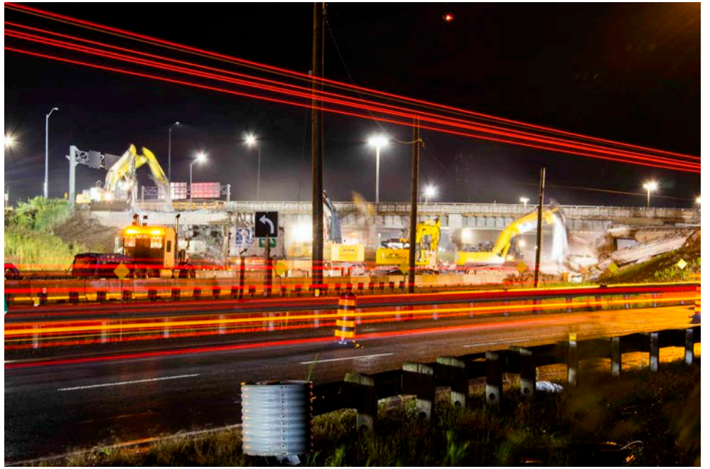
The old Glendale overpass is torn down by heavy machinery to make way for the newly completed diamond diverging interchange. Richard Harley is there in the early hours of the morning to capture the shot as cars are diverted around the construction.
