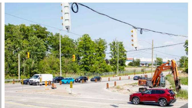
Construction of the roundabout at the Glendale Avenue and York Road intersection began this week and should be completed by the end of July. SOMER SLOBODIAN
