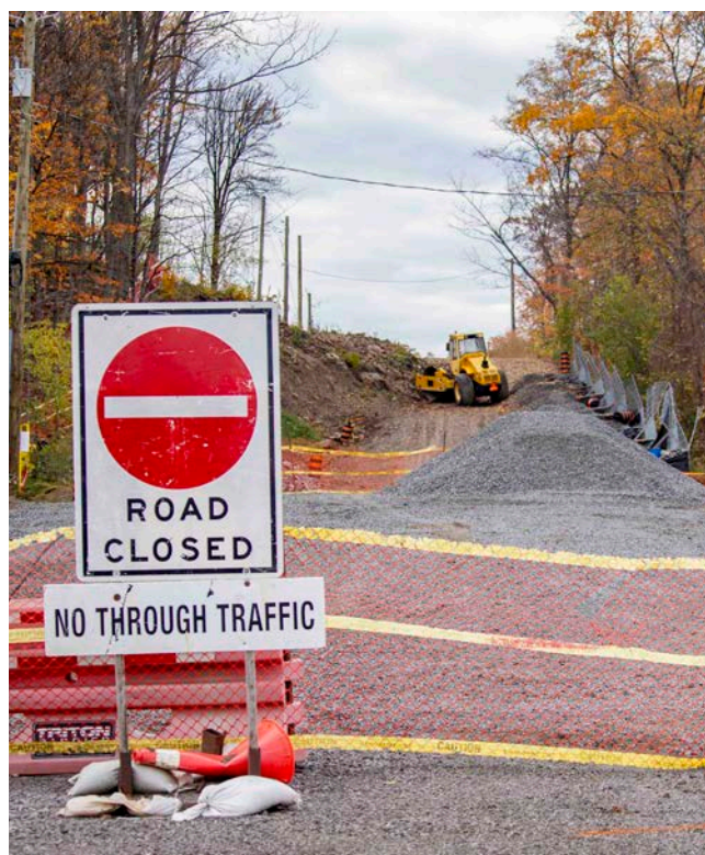
The $1.6-million construction project on Mewburn Road has resumed after an August snag stalled work. EVAN LOREE
