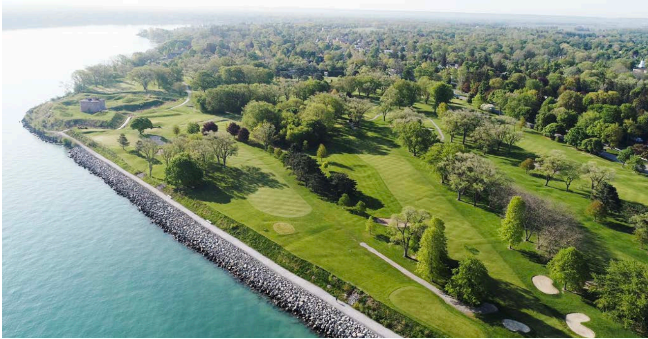
Parks Canada is constructing a 500-metre breakwall near Fort Mississauga. The project is expected to take about two years to complete and will require the removal of trees along the bank. RENE BERTSCHI/SKYVIEW ARTS
