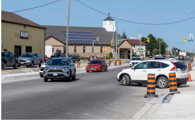
Construction continues to slow traffic on Niagara Stone Road in Virgil. But letter writer Susanne Langdon says it's nothing to have a conniption fit about. FILE PHOTO
