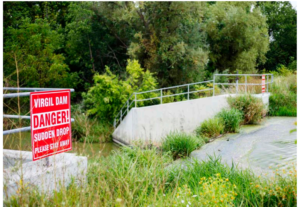
This dam, one of two in Virgil on Four Mile Creek, could be removed if the town is unable to reach an agreement with the Niagara Peninsula Conservation Authority on who will foot the half a million dollar bill for its required maintenance. EVAN LOREE
