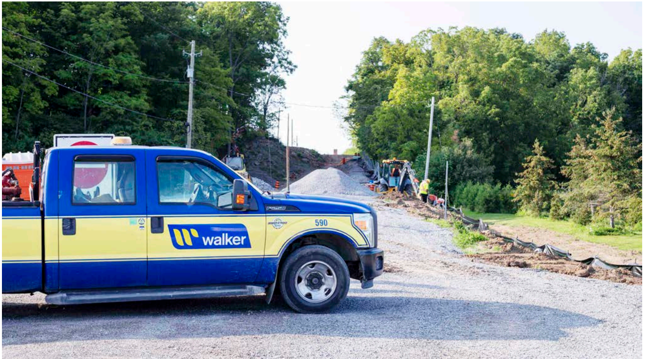
Construction on Concession 6-Mewburn Road has been delayed due to problems discovered by the contractor. EVAN LOREE
