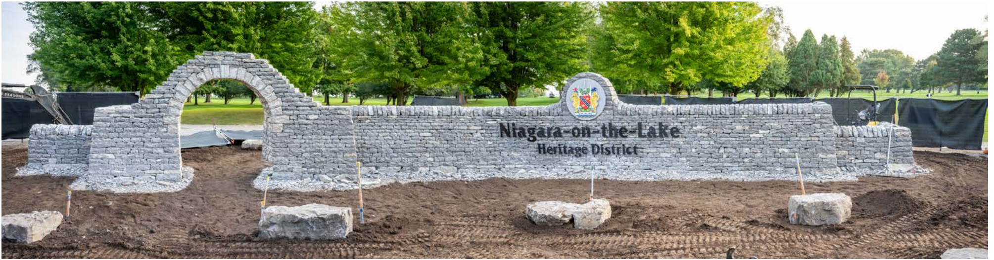
Niagara-on-the-Lake's new gateway wall at Mississauga and Queen is well on its way to being ready for a formal unveiling by the town. DAVE VAN DE LAAR
