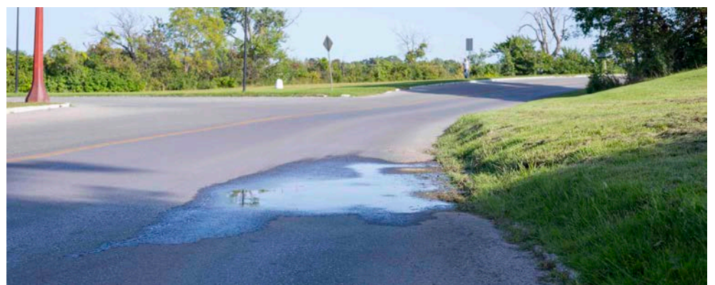
This innocuous spot of ground is always wet because there's a natural spring running underneath the Fort George grounds. EVAN LOREE
