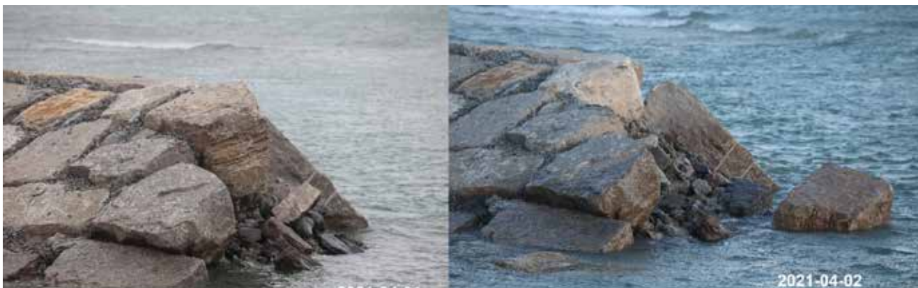
These two images by Ron Simkus show some of the damage the massive stone groyne has sustained. SUPPLIED
