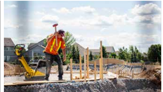
Steve Hare, president of Propour Concrete Services works on the new Virgil skatepark. RICHARD HARLEY
