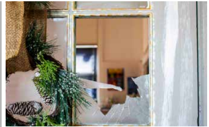
Broken windows can be found all over the old Virgil school. RICHARD HARLEY
