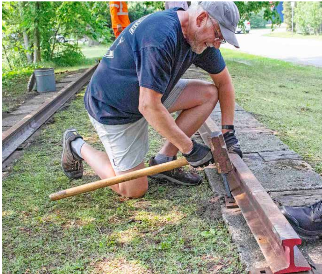
Dock area resident Ron Simkus bangs in a railway spike at a new display to commemorate an old stop. EVAN SAUNDERS
