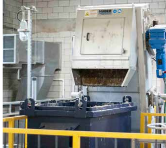
A mechanical bar screen removes incoming large debris, or “rags” from the sewage. BRITTANY CARTER
