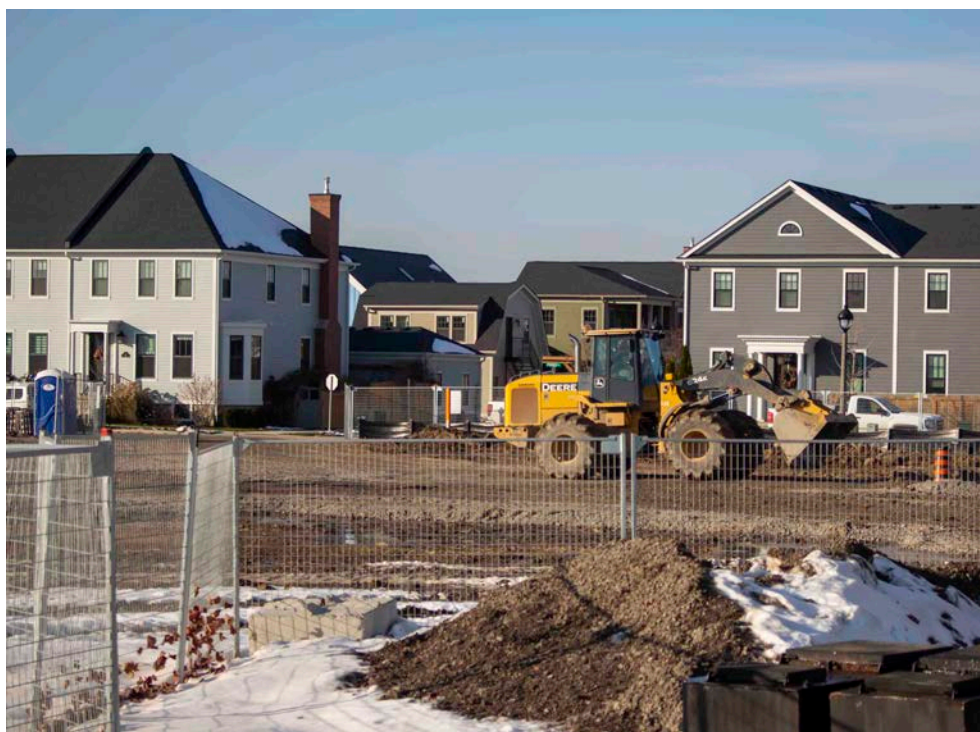
Preliminary work has begun on the expansion of the Village commercial development. Letter writer Jackie Bonic wants to see a specialty grocery store included. SUPPLIED
