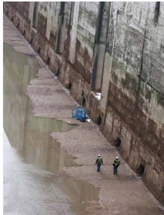
The canal's dewatering allows to inspect and repair the canal's infrastructure that is usually inaccessible during a navigation season. More photos at niagaranow.com DARIYA BAIGUZHIYEVA
