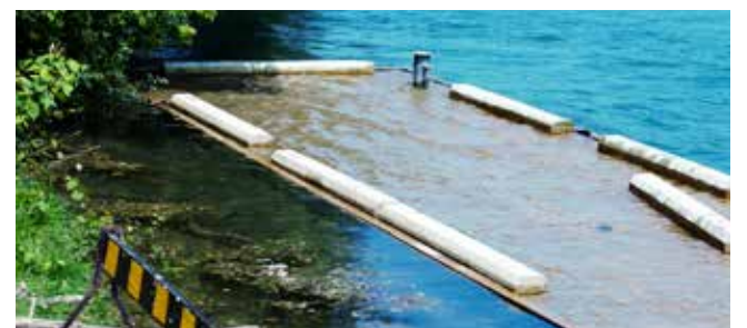
The dock at Navy Hall is almost completely submerged due to high water levels. BRITTANY CARTER
