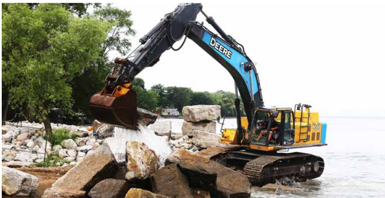
A failed rock groyne at Ball's Beach was repaired during the weekend. RON SIMKUS
