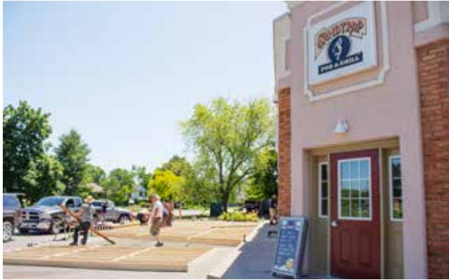
The Sandtrap Pub & Grill on Mary Street is building a new patio in its parking lot. JESSICA MAXWELL
