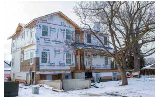
The house at 560 Missisagua St. where the fall occurred.
