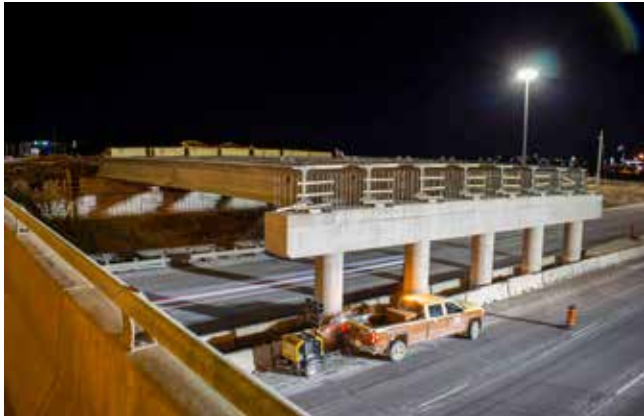
A crane was used to lift steel girders onto the new bridge on Monday and Tuesday nights. RICHARD HARLEY
