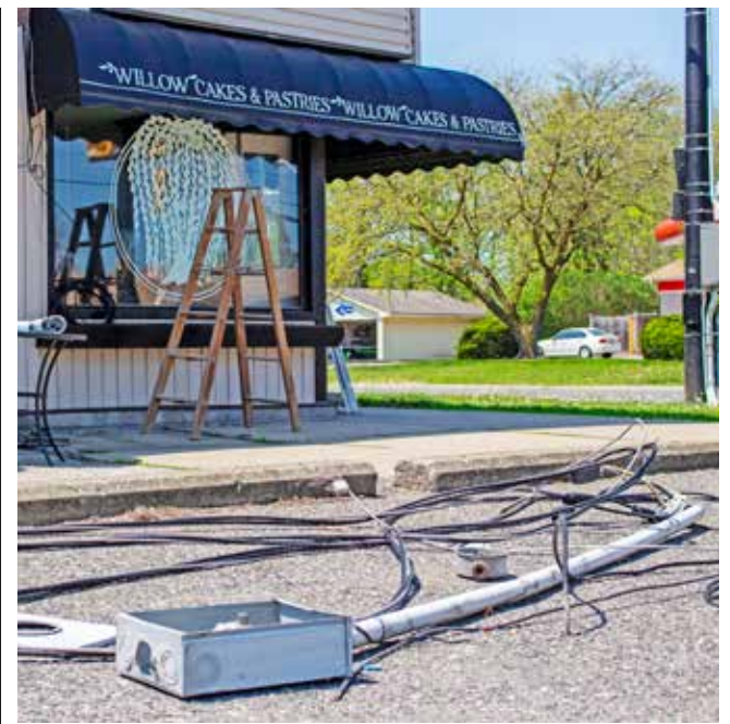
Electrical lines on the ground outside of Willow Cakes & Pastries after being pulled out of the building by a passing truck. JESSICA MAXWELL
