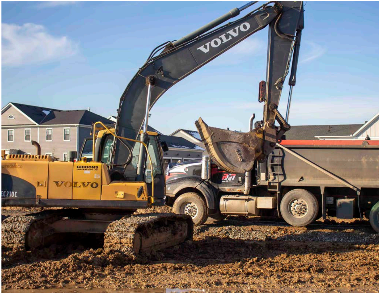
Heavy machinery digs up the earth in preparation for the next stage of the Village development. EVAN LOREE
