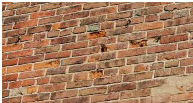
Spalling in Historical Brick Field. SUPPLIED
