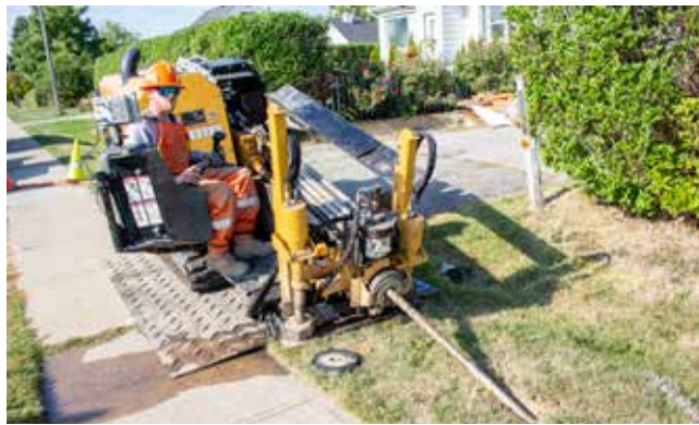
Ryan Bates operates the directional drill used to clear a path for the Fibe lines. RICHARD HARLEY
