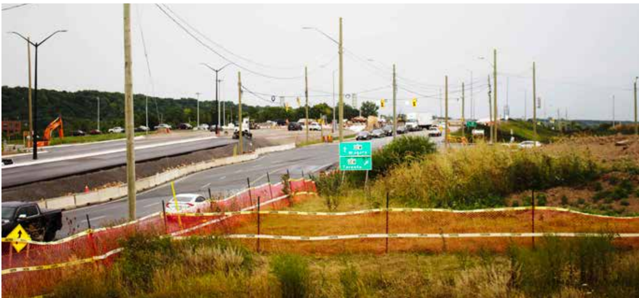
Work is nearing completion on the QEW’s new diverging diamond interchange at Glendale Road. EVAN LOREE
