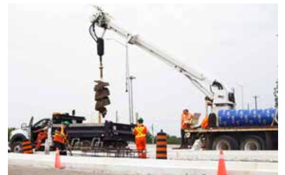
Construction crews work on the interchange, which will be open for traffic soon. EVAN LOREE
