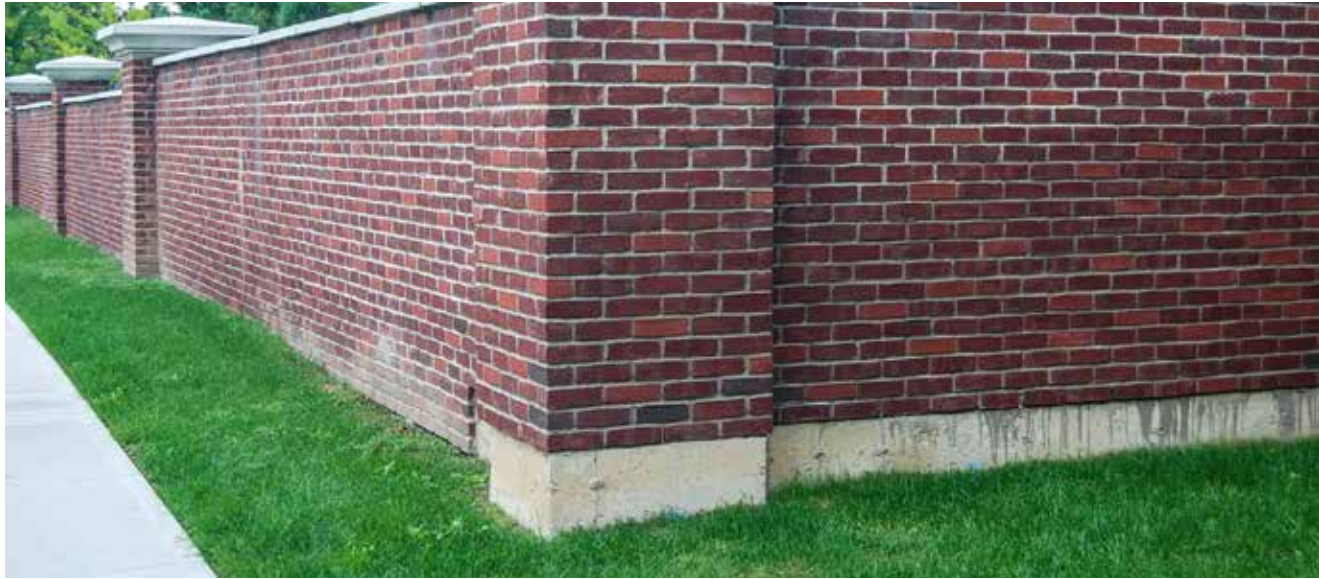
The case of the disappearing foundation. SUPPLIED/BRIAN MARSHALL.
