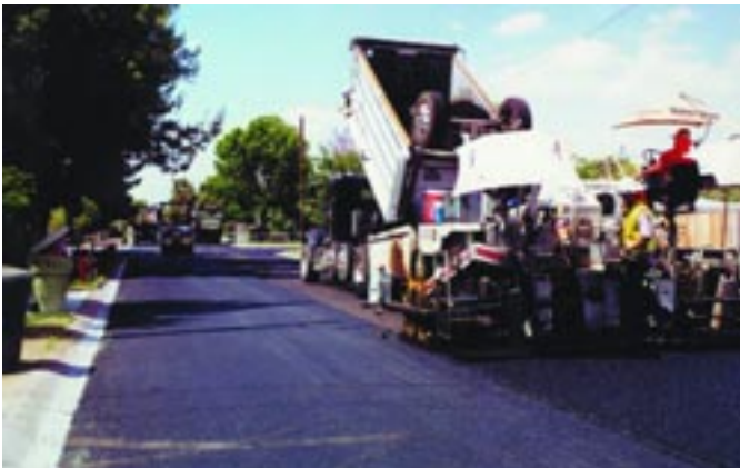
A paving crew from FNF Construction adds a thin asphalt-rubber overlay on a residential street in Phoenix in the summer of 2000, using the same paving equipment as that used to lay conventional asphalt.
