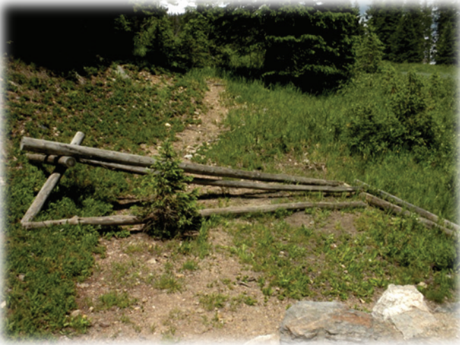
Collapsed Fence at Lake Irene, © 2015 Jonathan V. L. Kiser.
