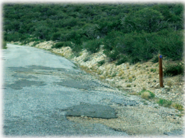
Wheeler Peak Drive Infrastructure Decay, © 2015 Jonathan V. L. Kiser.
