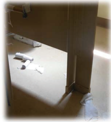
Bathroom Neglect, YNP Visitor Center, © 2015 Jonathan V. L. Kiser.
