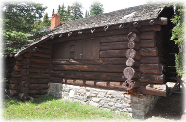
Lake Irene Chimney Infrastructure Issue, © 2015 Jonathan V. L. Kiser.
