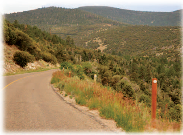
Safety Guardrails Lacking in GBNP, © 2015 Jonathan V. L. Kiser.
