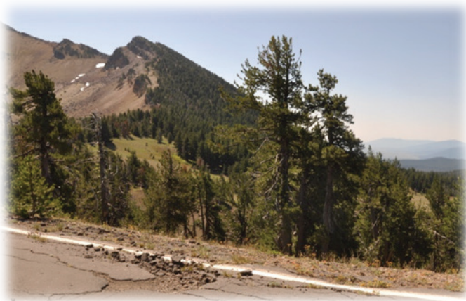
East Rim Drive Infrastructure Decay, © 2015 Jonathan V. L. Kiser.
