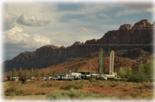
Fracking Operation in Moab, UT South of ANP, © 2015 Jonathan V. L. Kiser.
