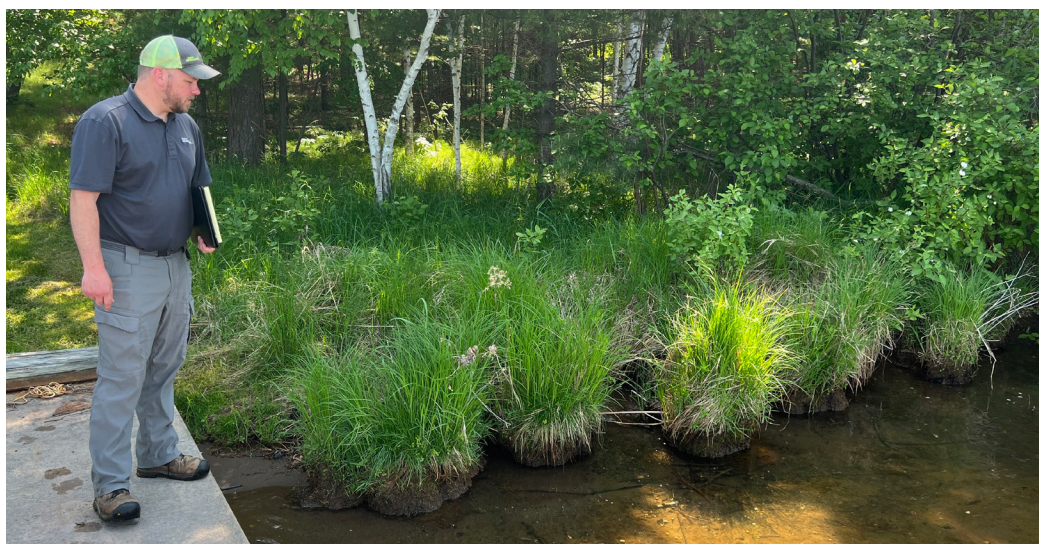
Shoreline loss caused by wave action needing remediation
