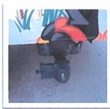
Liquid Waste Connection
