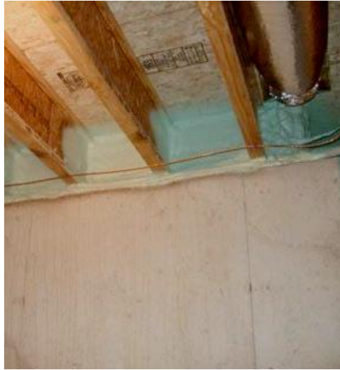
Above: Spray foam along the basement rim joist to provide a complete air barrier connecting the foundation wall, sill plate, rim joist and subfloor (Source: BSC, 2009).
