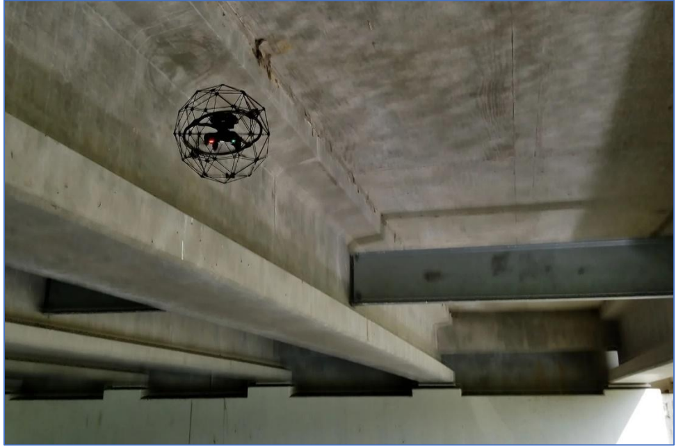
Figure 49 - So-called "indoor drones" can be used to perform infrastructure surveys in areas difficult for people to access.
