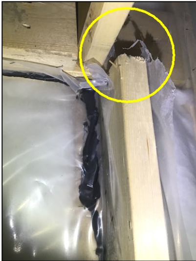
Stud not attached at joist. Recommend further review
