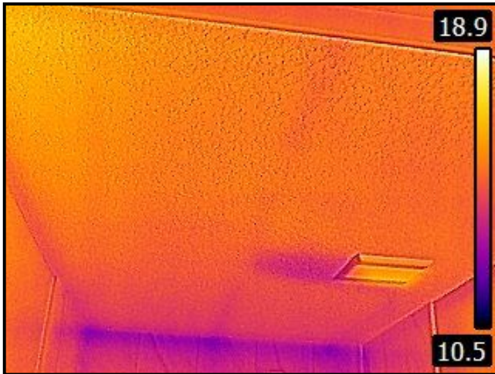
Upper Level Bathroom ceiling dry on Thermal scan
