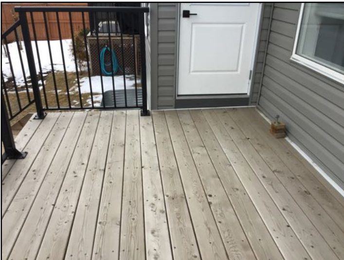
Deck in serviceable condition - On going maintenance suggested. Monitor all wood to soil contact for deterioration and address as and when required.
