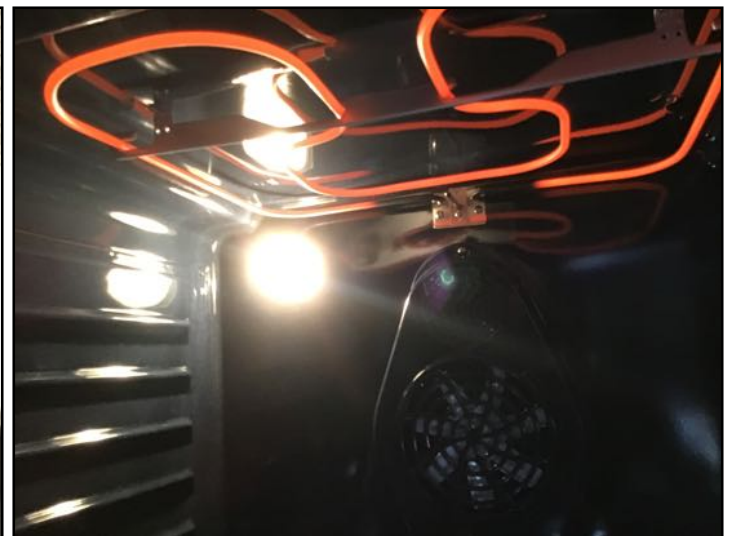
The electric oven broil element tested at the time of inspection and appeared to function properly. These can fail at anytime without warning. No guarantee, or certification is given as to future failures.
