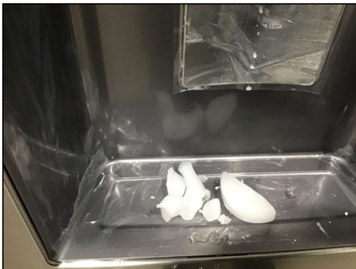
Ice maker tested and worked on the day of the inspection
