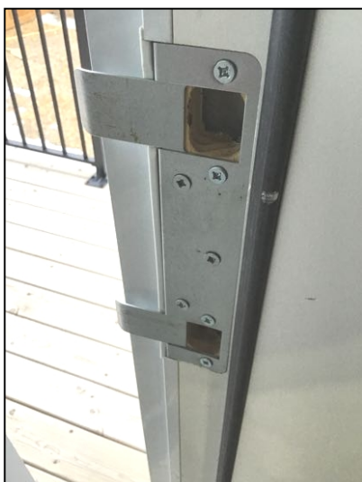
Recommend striker plate adjustments to ensure snug fitting door at weatherstripping.
