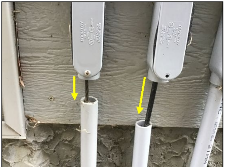
Conduit has pulled away from box. Recommend repairs as required.
