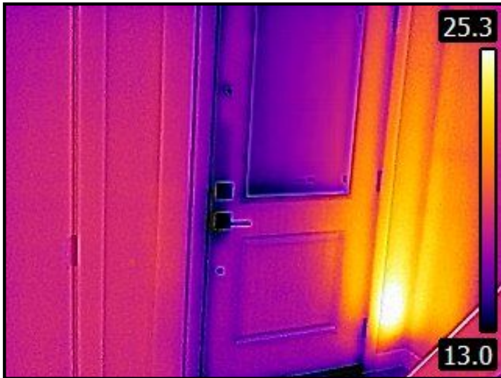
Front Entryway - Thermal Image
