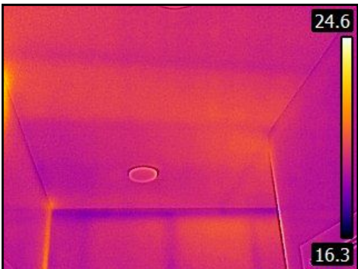
Mud Room ceiling thermal scanned and no major causes for concern noted.
