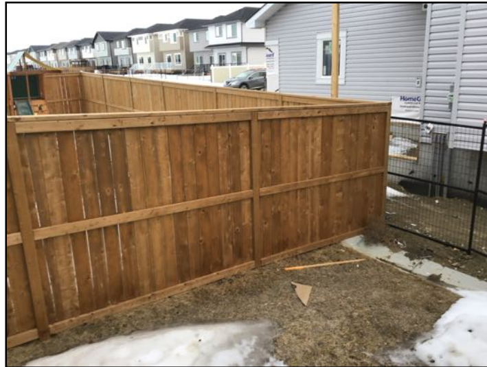
The fence is in serviceable condition. Sealing external wood as required will prolong its life span
