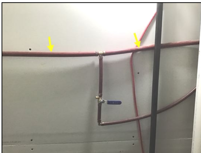
Loose hanging supply line. Recommend securing.
