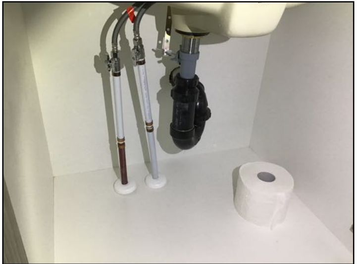
No leaks observed at the Upper Level Bathroom sink during the inspection
