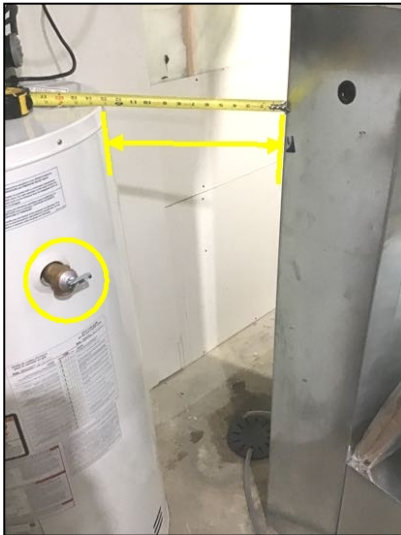
Caution: Limited access space to Furnace / Service Panel. Avoid disturbing TPR valve for safety
