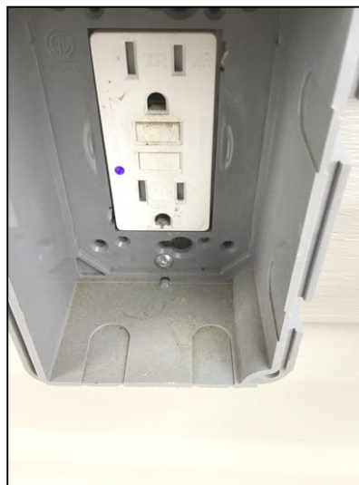
GFCI in place and operational
