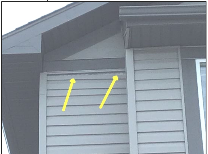
Gaps noted in vinyl siding. Recommend adjusting to prevent possible water entry.
