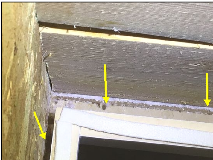
Recommend insulating gaps between hatch lip and curb to prevent heat loss and staining
