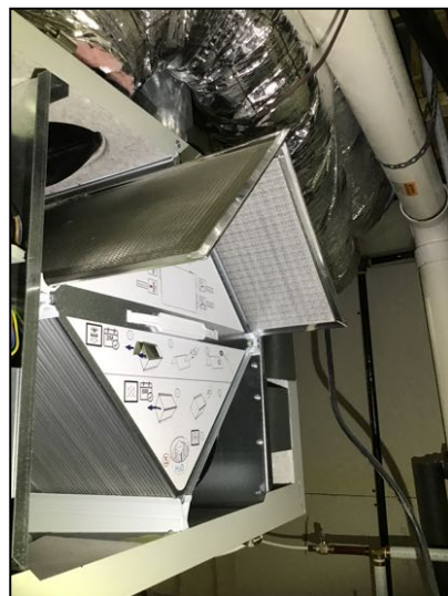
Recommend cleaning HRV filters and core regularly.
