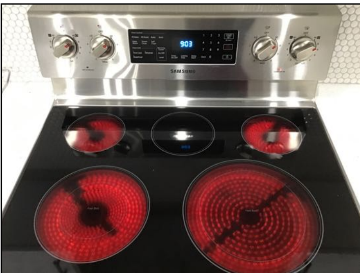
The electrical stove elements were tested at the time of inspection and appeared to function properly. These can fail at anytime without warning. No guarantee, or certification is given as to future failure.
