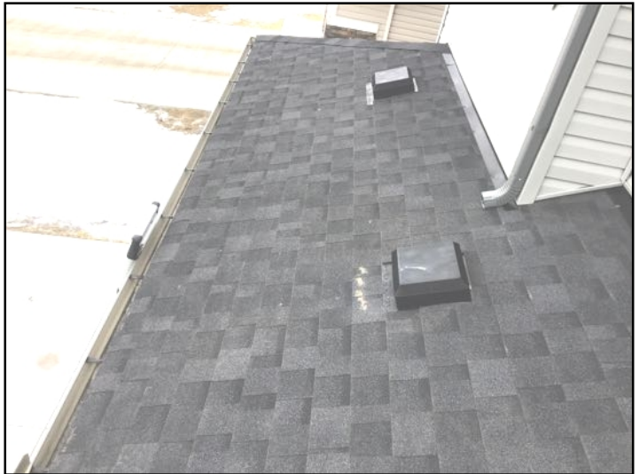
Garage roof is in serviceable condition where visible. Comments made on the condition of roof are made on the day of the inspection only - a claim cannot be made for any deficiency after the inspection date.
