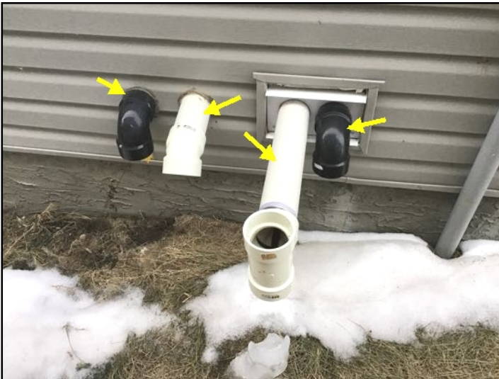
Loose venting noted. Secure to prevent damage
