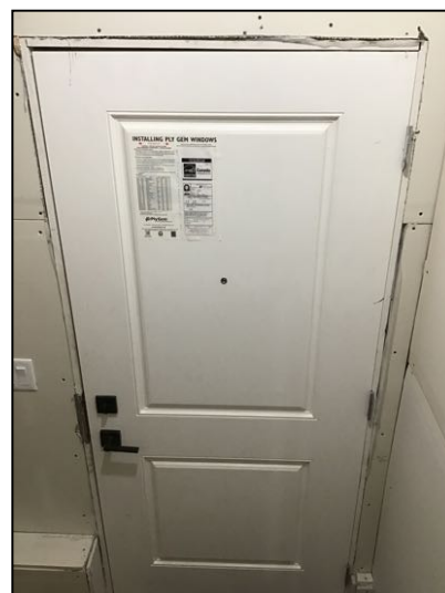
Side entryway door sticks and requires adjustments for smooth operation.
