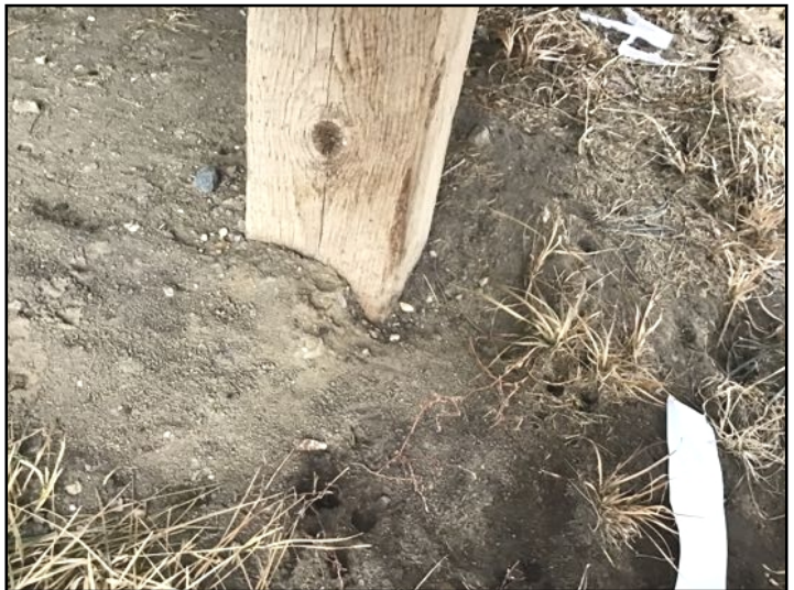
Unable to fully review the structure of the deck. Framing appears sturdy and secure but comments are limited due to this. Difficult to determine depth of support posts. Insufficient depth of concrete piers can result in heaving due to frost. Recommend further review of deck components by qualified contractor if a more invasive inspection is required.
