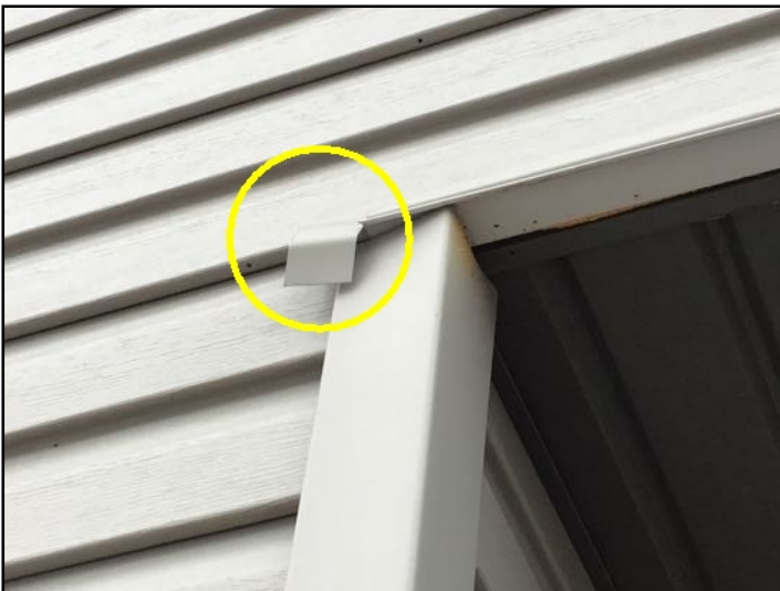
Tag noted at siding. Recommend further review
