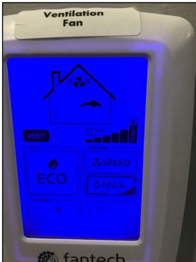
HRV control panel
