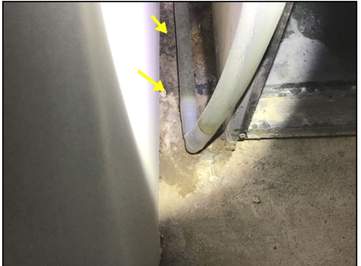
Active condensate leak noted at high efficiency furnace drain line - Repair asap to prevent long term damage to furnace.
