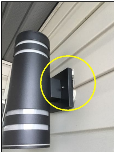
Loose light fixture(s) observed. Recommend securing for safety.
