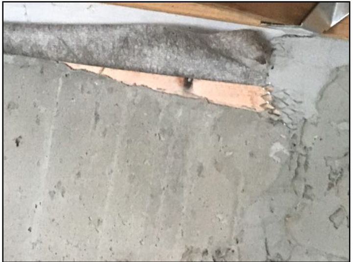
Recommend sealing exposed rim joist
