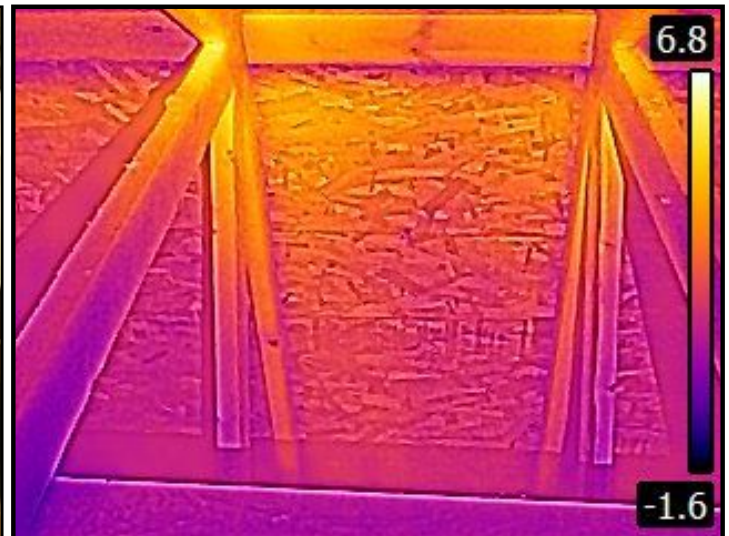
The sheathing was thermal scanned and appeared dry on the day of the inspection
