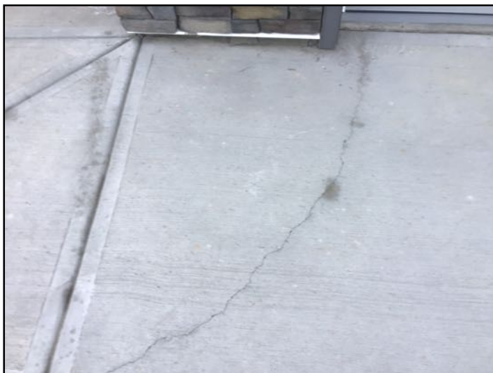
Cracking noted on driveway
