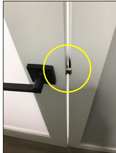
Kitchen pantry door does not latch.
