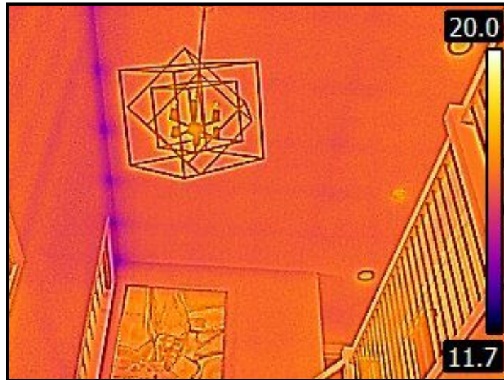
Upper Stairwell ceiling thermal scanned and appears dry on the day of the inspection.
