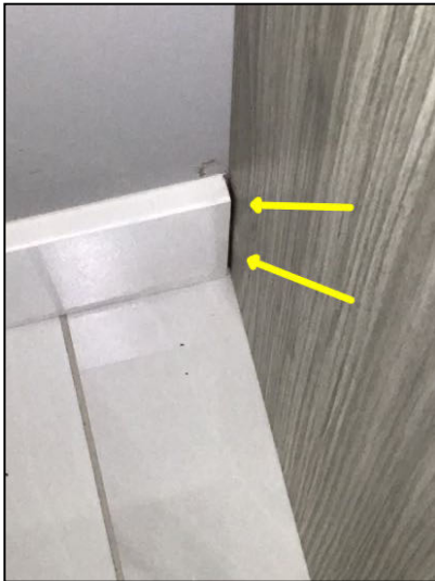
Recommend sealing all gaps to prevent water damage.
