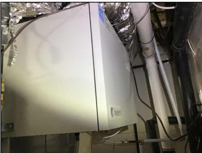
HRV (Heat Recovery Ventilation) system in place - These systems contain filters that require regular cleaning. Suggest maintaining as per manufactures recommendations.
