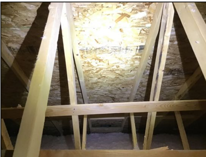
The sheathing was visually inspected and appeared dry on the day of the inspection. (we can only comment on what is visible and accessible areas from the attic hatch at the ladders edge)
