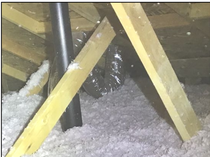
Recommend further review of bathroom exhaust venting. Loop can hold water which in turn can freeze.
