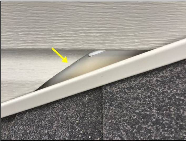
Areas of siding cut poorly in areas.
