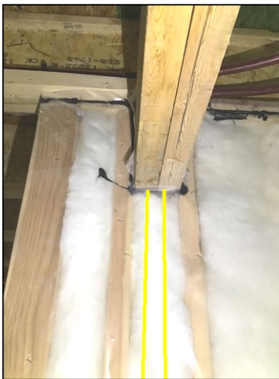
Unable to review beam ends. Recommend installing additional support
