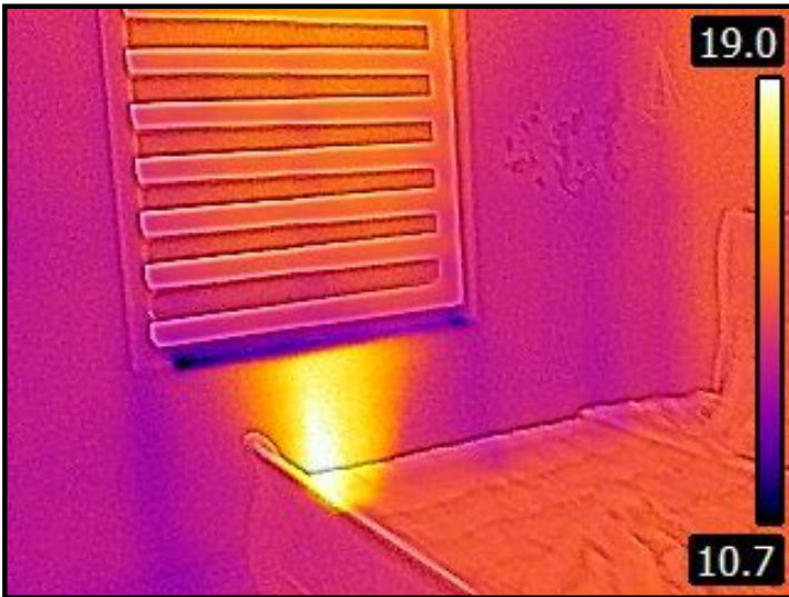
Bedroom 3 - Thermal Image - Walls and ceilings thermal scanned. No major causes of concern where visible.
