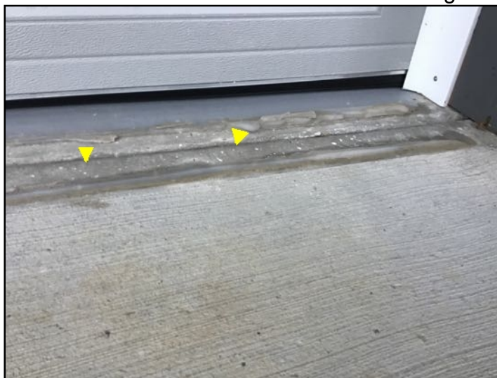
Slight settlement noted at driveway slab.
