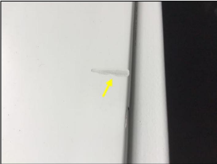
Damaged noted at Bedroom 2 window sill.
