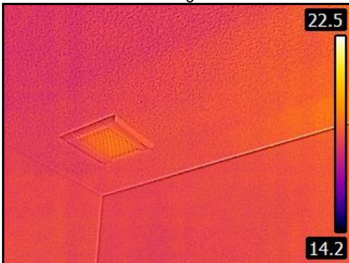
Main Bathroom ceiling dry on Thermal scan
