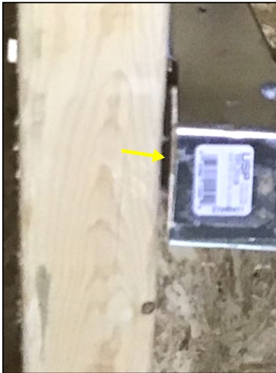
Joists have separated in areas.
