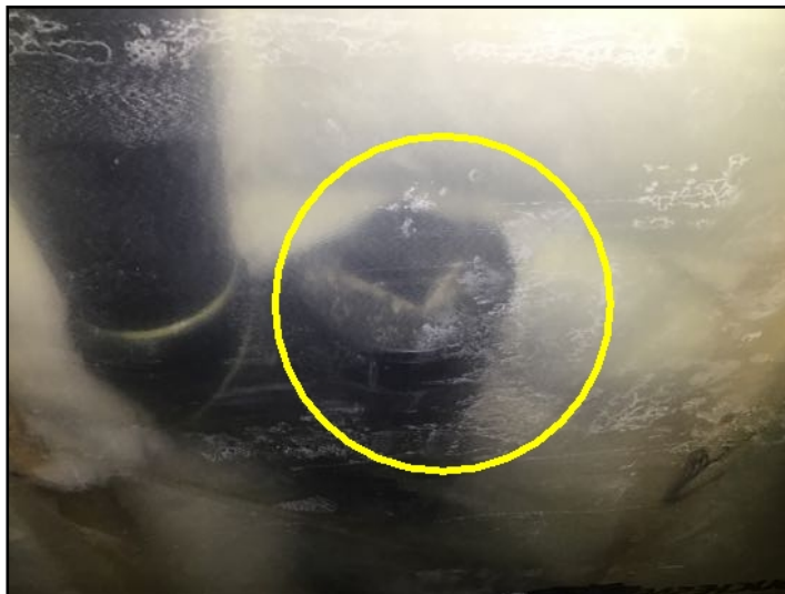
Clean out observed
