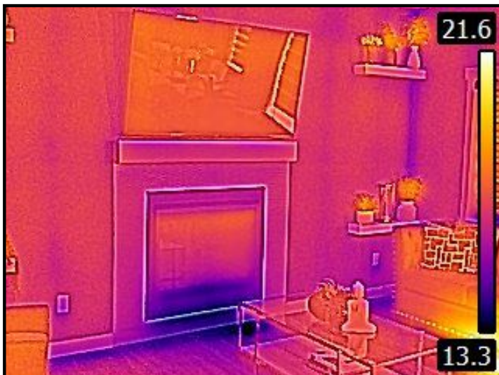
Living Room - Thermal Image
