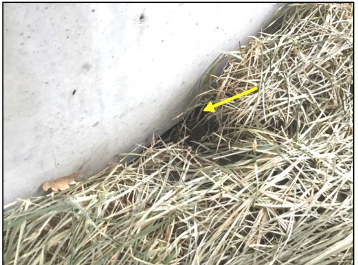
Negative grade / void observed under porch. Recommend back filling to prevent water pooling at foundation wall and to prevent animal intrusion.
