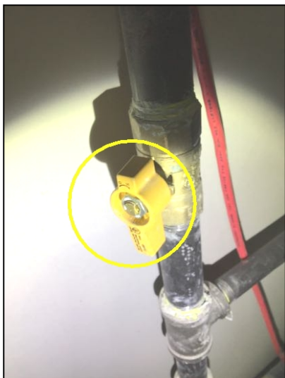
Gas shut off
