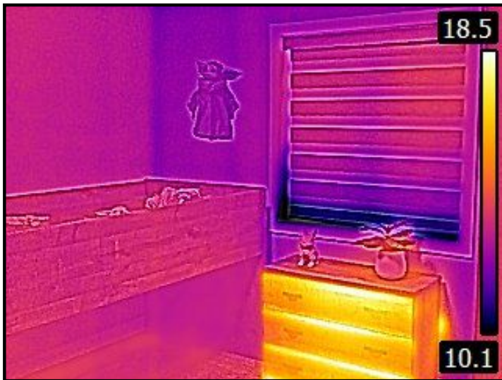
Bedroom 2 - Thermal Image - Walls and ceilings thermal scanned. No major causes of concern where visible.
