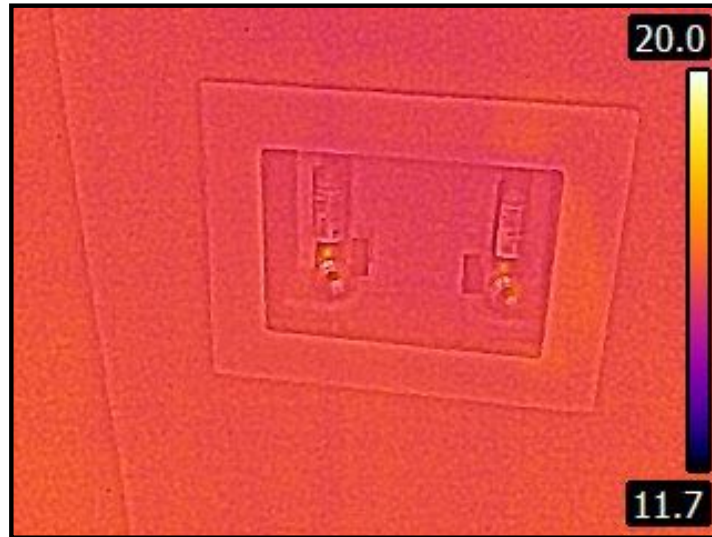
Washer supply scanned for leaks - no issues to report
