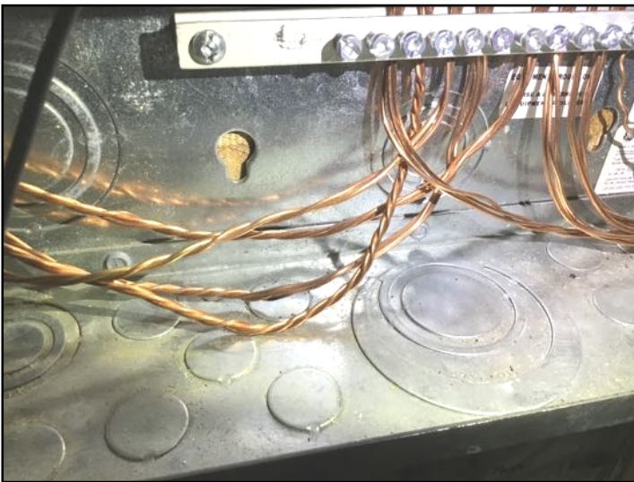
Copper wiring observed at the main panel
