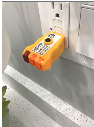
GFCI in place and operational in Upper Bathrooms.
