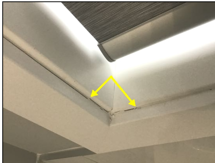
Peeling paint / split caulking observed. Repair as required.
