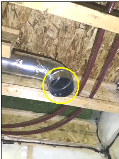
Missing diffuser noted. Replace as required
