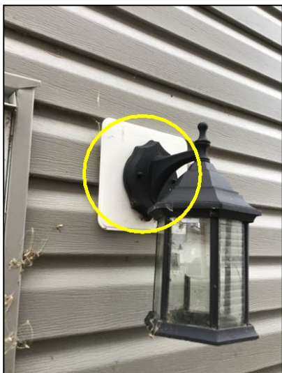
Secure loose light fixtures for safety.
