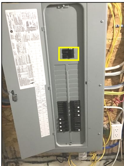
Main disconnect switch shown - 100 Amp
