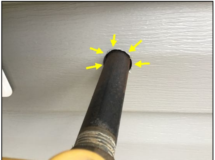
Suggest sealing/caulking all holes and gaps as part of routine maintenance.
