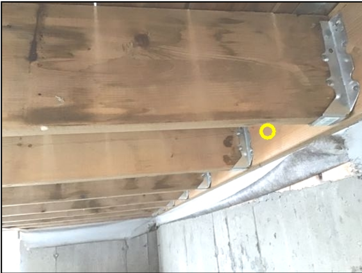
The ledger board is attached to the home with nails. Recommend upgrading to lag bolts for strength, particularly on raised decks
