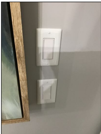
Recommend labelling fireplace switch to prevent accidental ignition.
