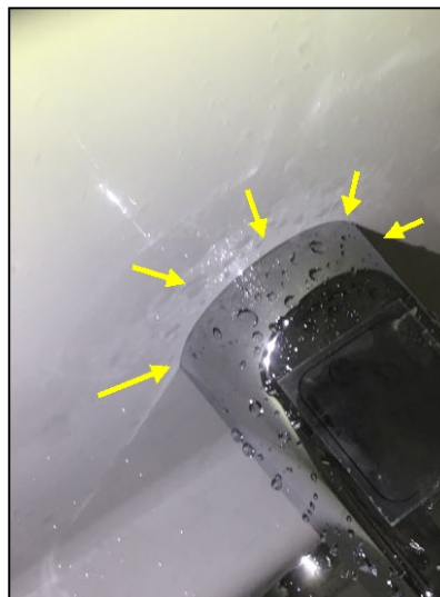
Recommend regular review of bathroom tub spout / wall gaps to prevent water damage to the wall behind. Re-apply sealant as required.
