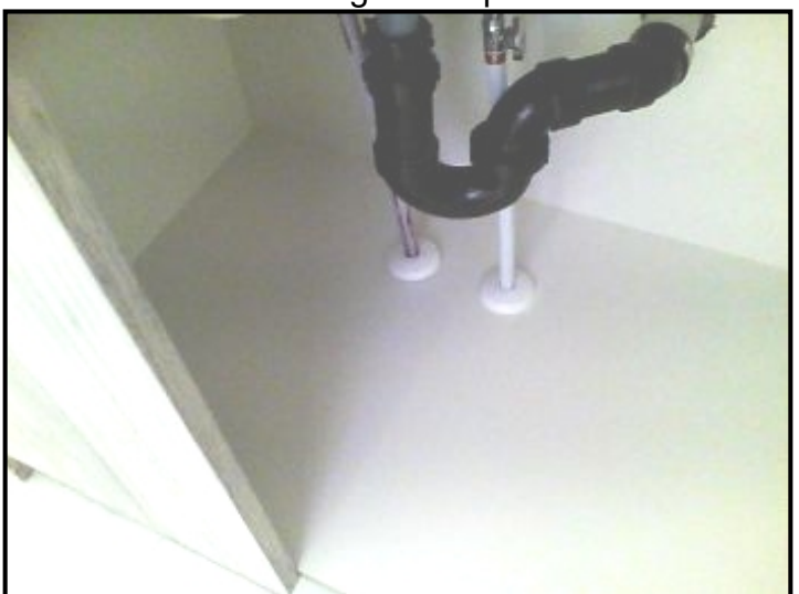
No leaks observed at the En Suite Bathroom sinks during the inspection
