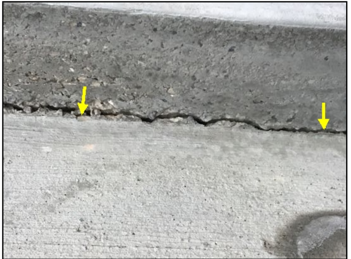
Walkway has settled in areas. Recommend repair as required
