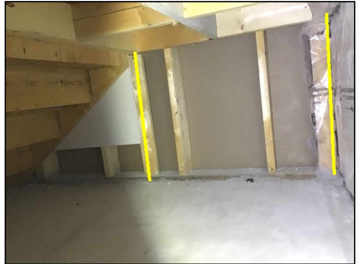
Recommend installing additional vertical posts beneath landing framing for additional support.
