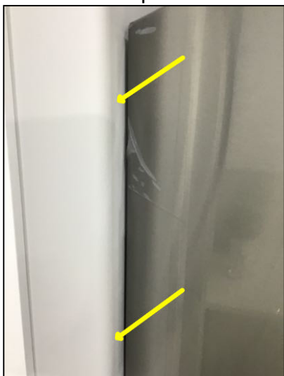
Left refrigerator door in contact with wall. Recommend repositioning refrigerator to prevent damage.
