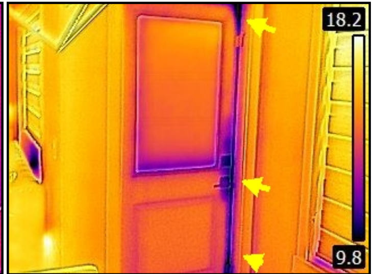
Rear Entryway - Thermal Image Cold drafts noted.
