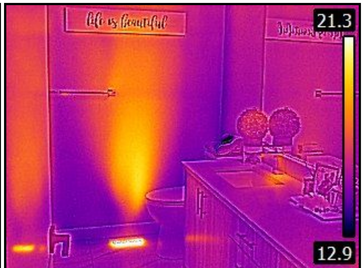
En Suite to Primary Bedroom - Thermal Image
