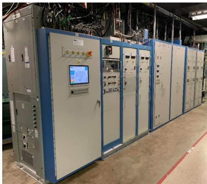
Fig. 1. L-Band radar transmitter group with (left to right) Controls Cabinet, Auxiliary Rack, HVPS 1 & 2, Capacitor Bank Cabinets (two) and Modulator Cabinet.
