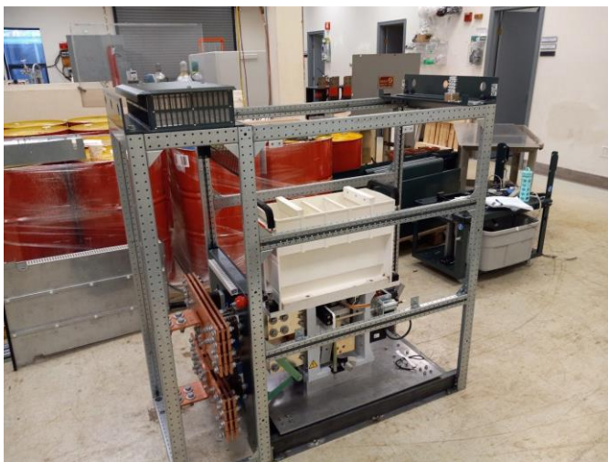
Fig. 5. DTI-modified hybrid circuit breaker with ruggedized, smaller enclosure. The cream-colored volume is the arc chutes. These will be removed and replaced with the hybrid semiconductor switch.
