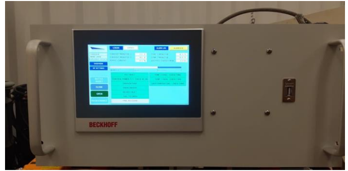
Fig. 6. Local SSCB controls. Unit may also be networked for coordinated switchgear operation.
