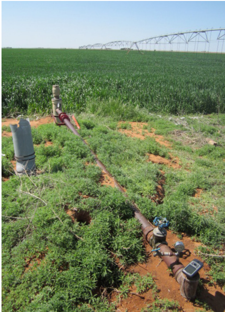
Irrigation well in Curry county, which supplies the center-pivot sprinkler sytem in the background.
