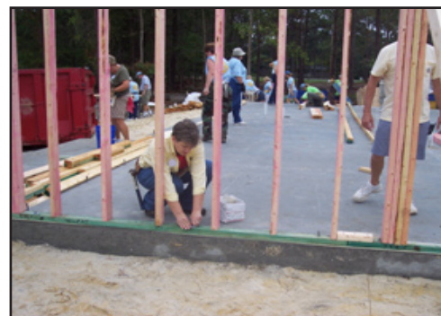
Kathy tightens bolts on new wall at North Myrtle Beach Women Build
