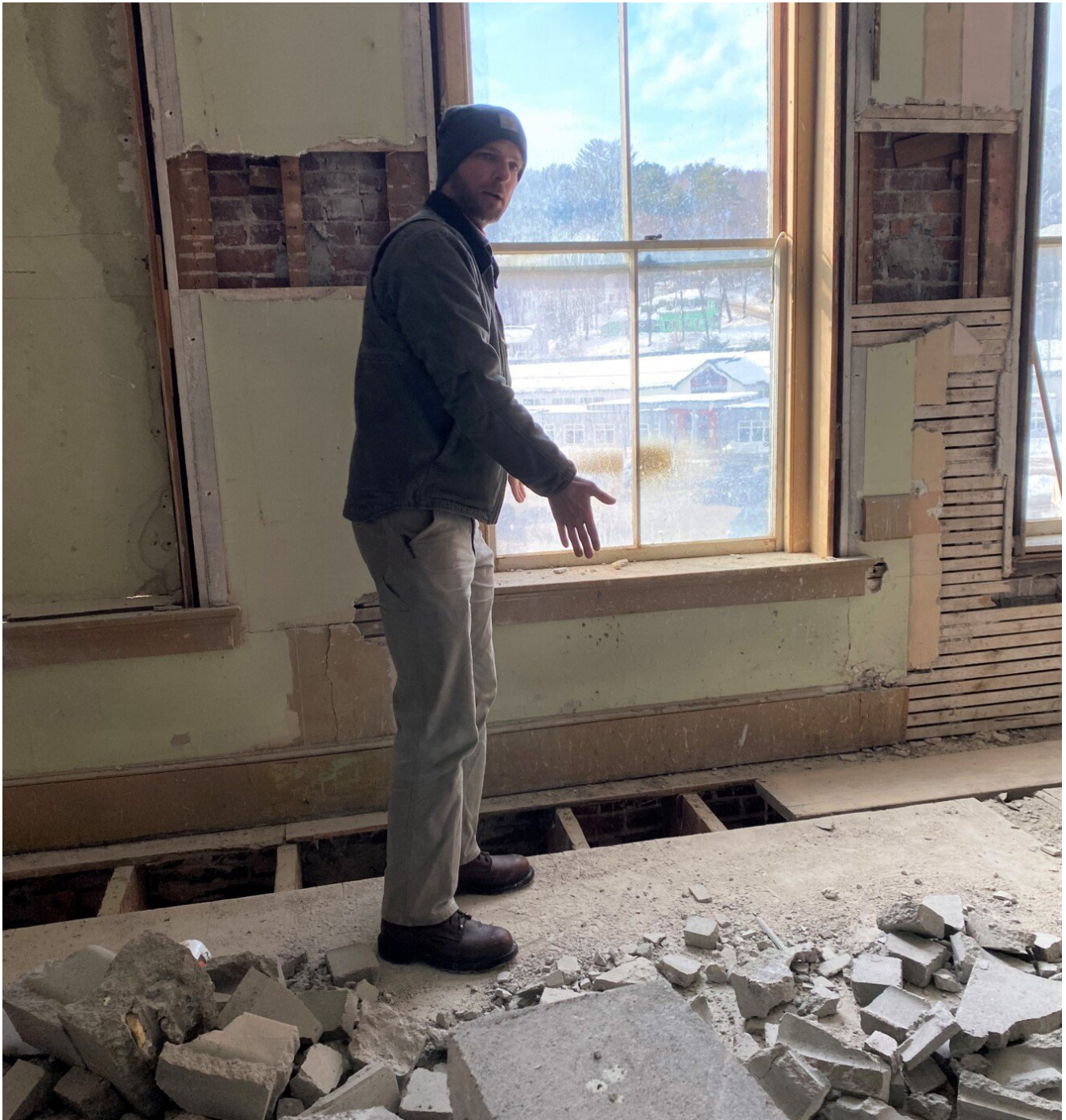
Mike Hanes, the developer who is transitioning the vacant Odd Fellows Hall into affordable housing, shows where makeshift block supports have been removed from the south side of the building wall and proper repairs will be made. Nicole Carter / Advertiser Democrat
