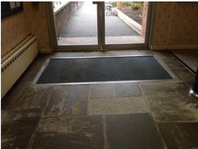
A33 _Tripping hazard and ADA issue at entrance walk-off mat pockets-replace mats
