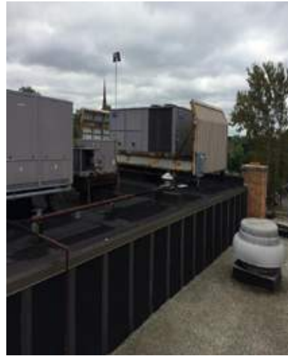
E2_RTU's on Roof
