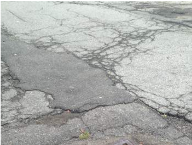
A14 _Gaston Street parking lot - mill and repave, restripe, proper ADA signs and layout
