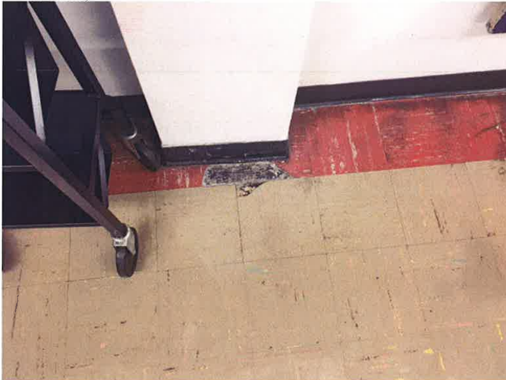
#4 – 1959 basement; 9x9" Tan & Red floor tile and Red tile mastic- confirmed as ACM
