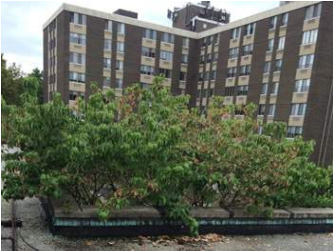
A9 _Trim trees overhanging the roof
