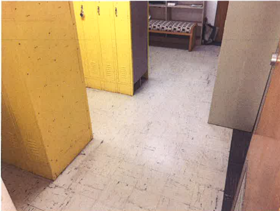
#6 – 1959 basement- 9x9” White floor tile confirmed as ACM
