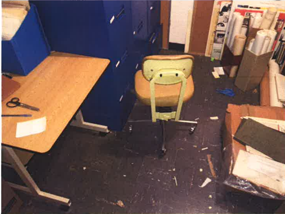
#5 – 1959 basement- 9x9” Grey floor tile and mastic- confirmed as ACM
