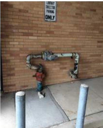
E5_Gas Service and Meter on Outside
