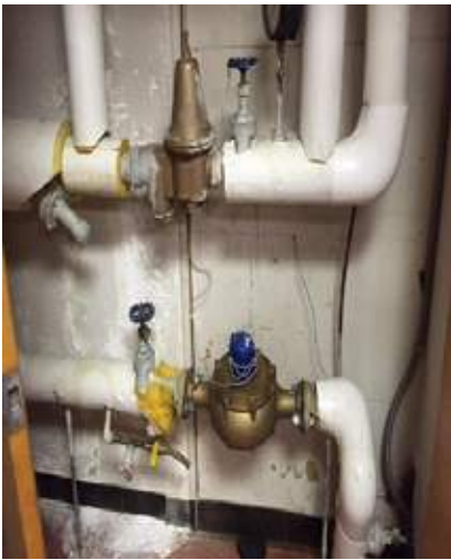
E3_Water Service , Meter and PRV
