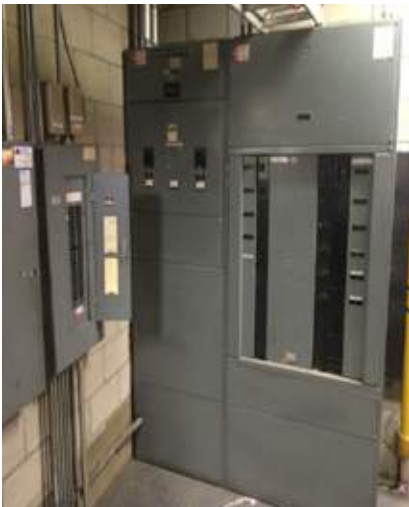
E9 _Building Service Switchboard-1978
