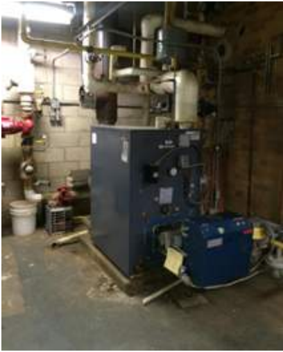
E1_Existing Boiler in Basement
