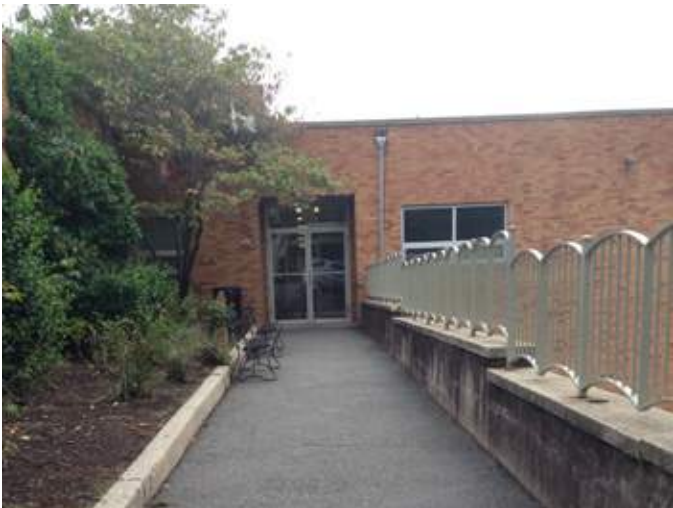
A8 _Trim trees overhanging the roof
