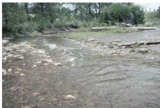
Above: This is a photo of the newly modified old stream channel after the project was completed.
