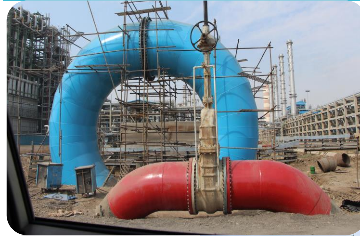
Fire Water line
