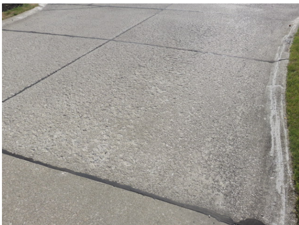
Isolated section of severe spall
