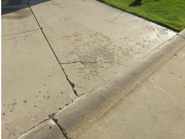
Cracks and spall at residential driveway (Homeowner responsibility for replacement)
