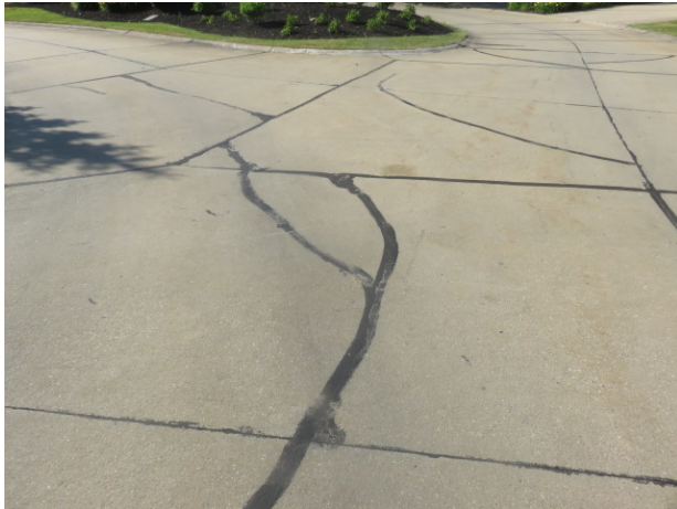
High frequency of repaired cracks at intersection
