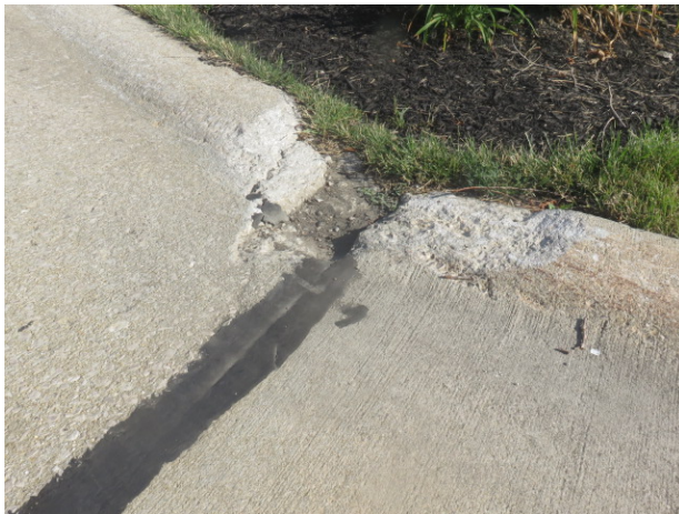
Chip at edge of street
