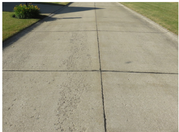
Isolated section of minor spall
