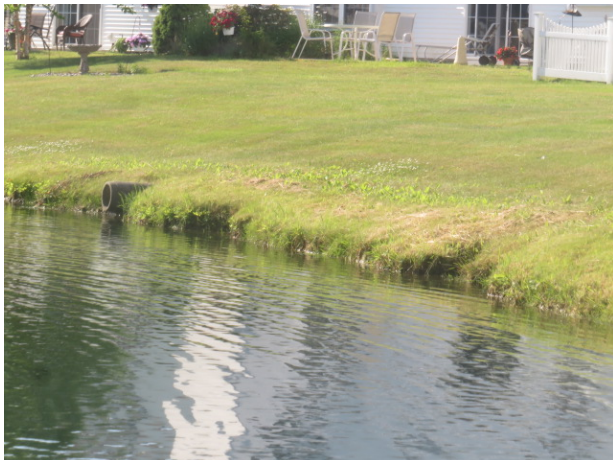
Shoreline erosion at east shoreline
