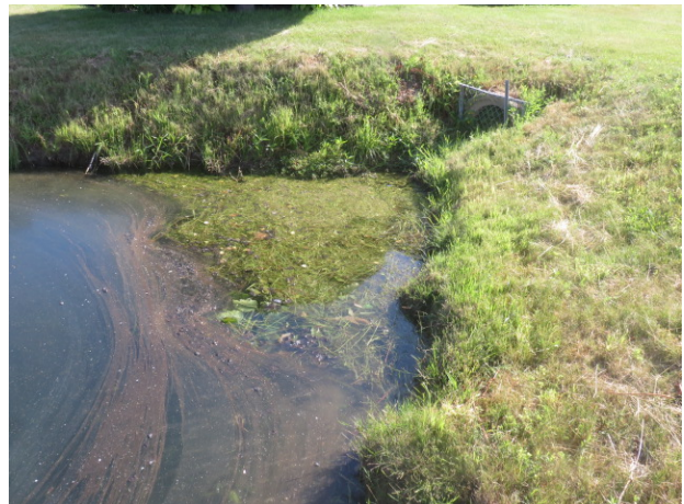
Shoreline erosion at east end of pond
