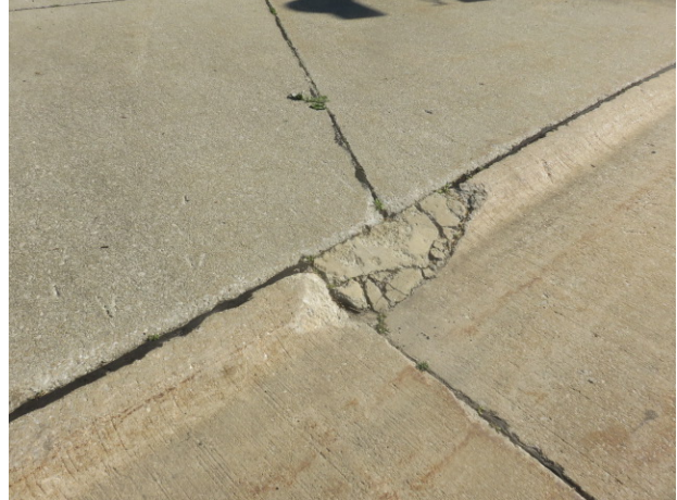
Deterioration at intersection of street and driveway
