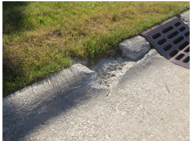
Large chip at street edge near catch basin
