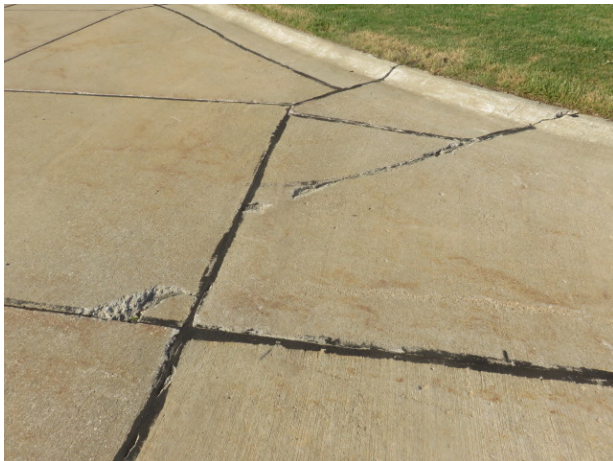
Cracks and chips at intersection
