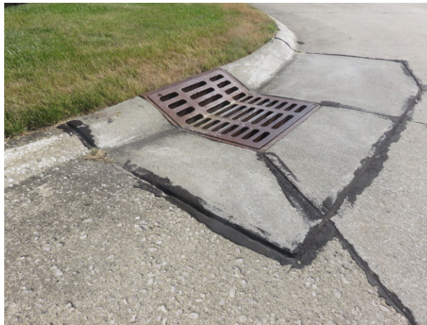
Concrete catch basin with metal grate
