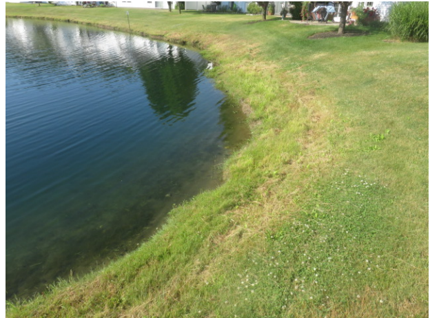
Minor erosion and loss of ground cover at west shoreline
