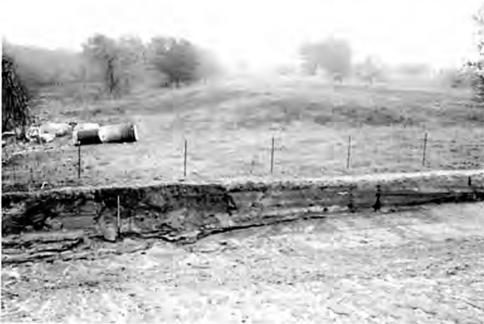
Figure 2. The right (south) bank of Smith Creek downstream from the Highway 119 crossing showing the prominent levee that was cut by road construction (note long-handled shovel and fence posts for scale).
