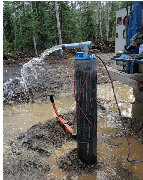
Well with a through the top setup.
