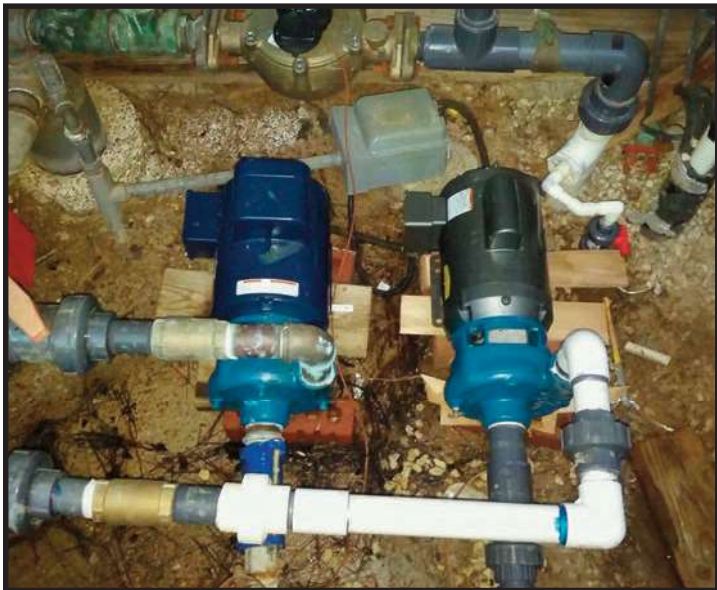
Booster Pumps Installed to keep our water pressure flowing
