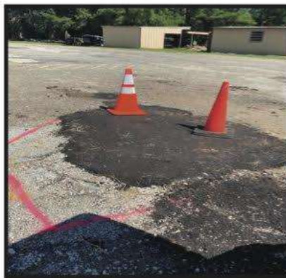
Potholes near clubhouse
