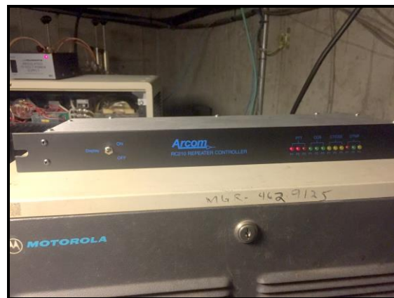
ARCOM AR210 Repeater Controller on top of the UHF linking MSF5000
