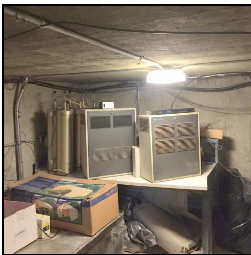
CARA Motorola MSF-5000 installation November 19, 2016 All Photo Credits – W1JGM
