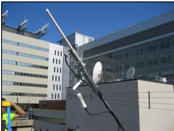
Fan dipole support bracket with Danbury Hospital back-up EMS antenna above.
