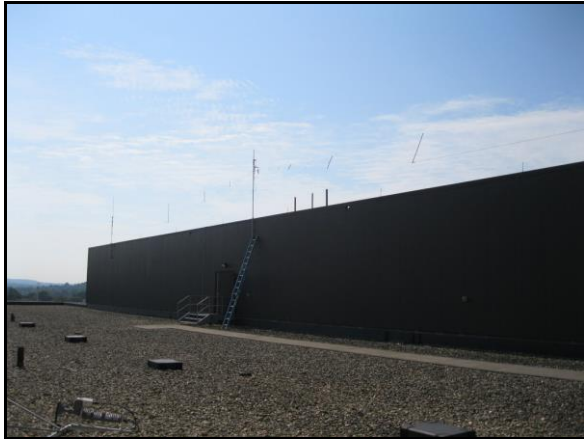
HF and VHF antennas: Danbury Hospital Strook Tower - penthouse mechanical room.
