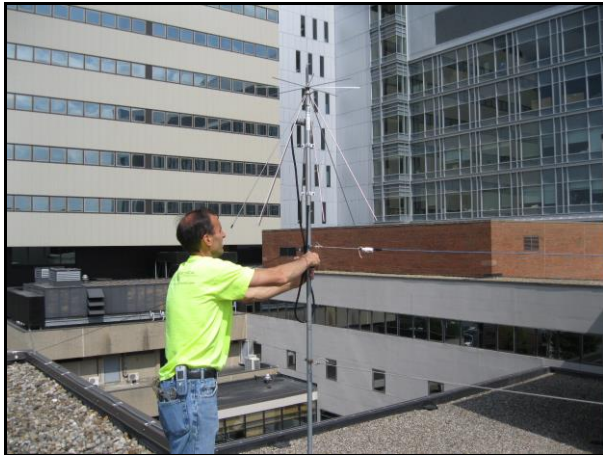
Perry Simone repairing the PL-259 connector on the Discone Antenna #2 attached to the Penthouse on the Strook Tower.
