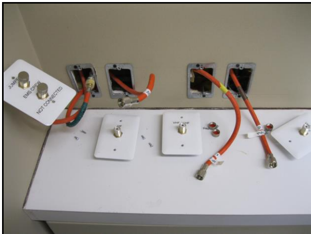
Checking and labelling conference room bulkhead connectors for the VHF and HF antennas.
