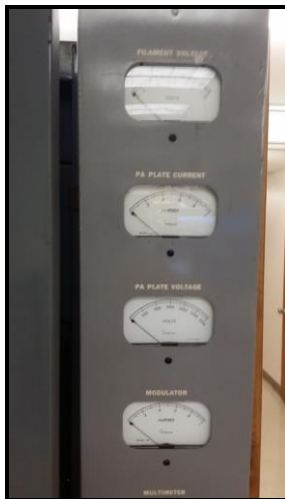
Full metering of all operating parameters is included.
