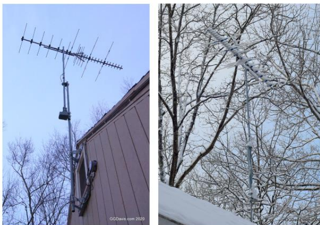
OVER THE AIR BROADCAST TELEVISION ANTENNA SYSTEM
