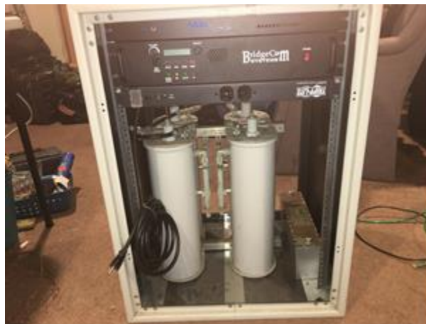
Front view of CARA's new 220 MHz. repeater rack
