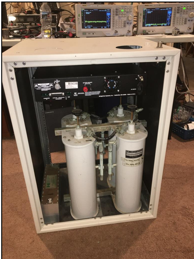
Rear view of CARA's new 220 MHz. repeater rack
